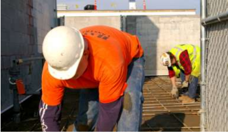
Construction workers set reinforcing bar to prepare to pour a concrete floor.
