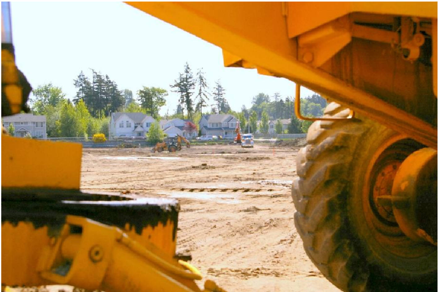
Earth-moving equipment prepares the ground for field improvements at Honey Dew Elementary School.
