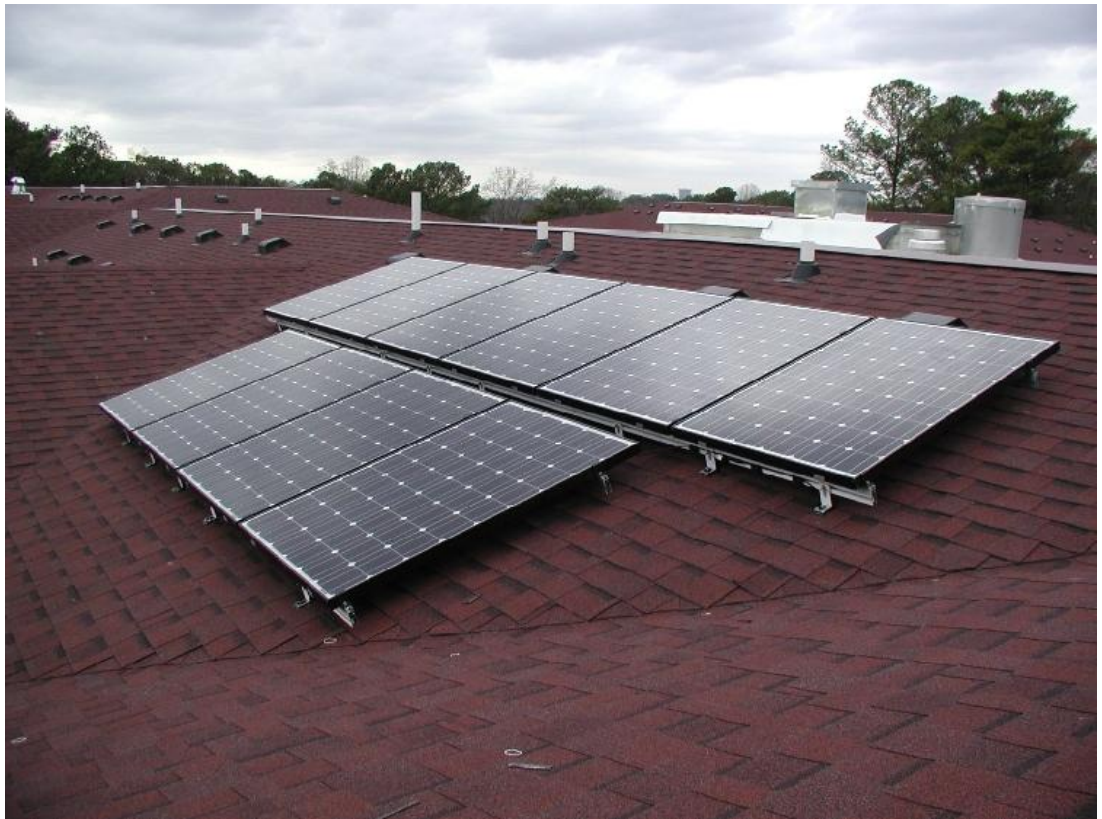
Hazen High School and Dimmitt Middle School soon will install solar panels (like those in the photo) as part of a renewable energy demonstration program with Puget Sound Energy and Seattle City Light.
